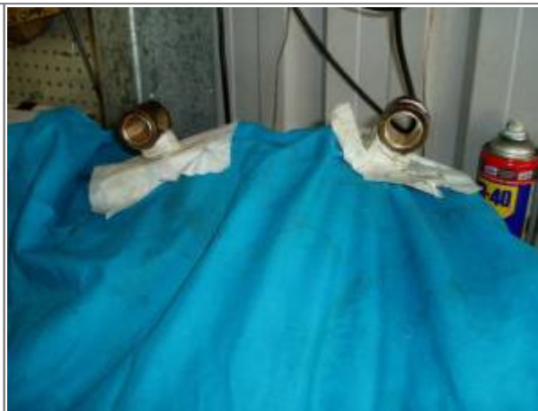
Two holes in a rag with some tape stops any bronze chips from getting down in the crankcase. 10)
