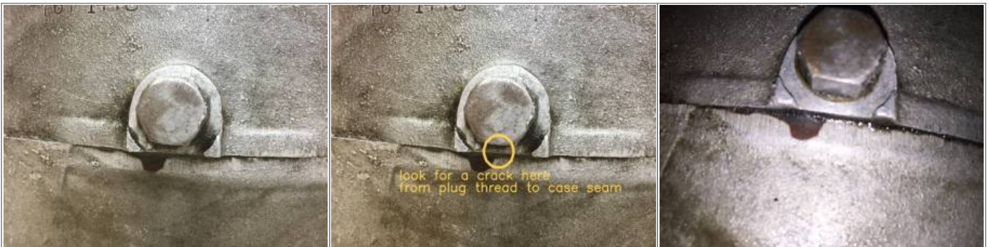
Leak around oil drain plug. 45) In this instance, the case seam appears to be weeping oil.
